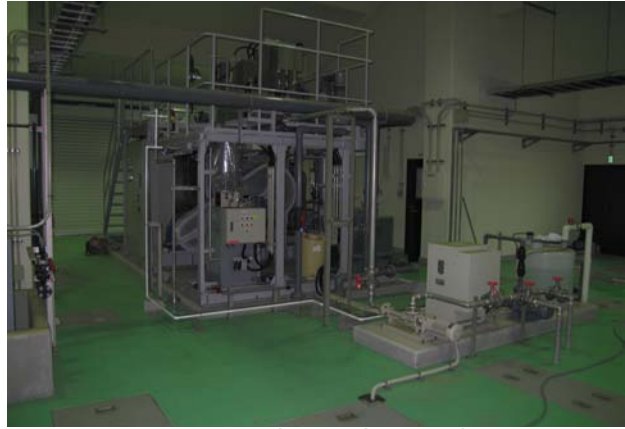
Namegata City Tamatsukuri North Regional Wastewater Treatment Plant (interior)
