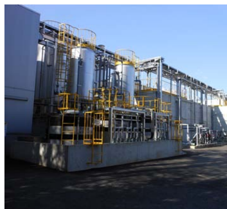
Effluent treatment facility
